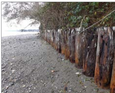
Eroding wood bulkhead (Photo: Scott Chase)
